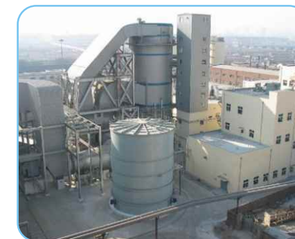
脱硫塔 Desulfurization tower
