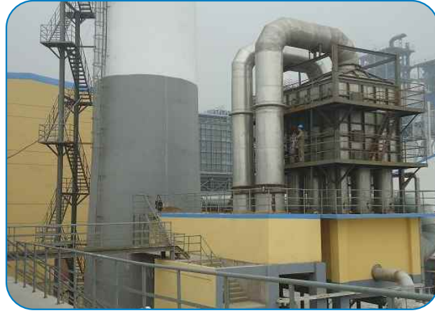
除尘设备 Dust removal equipment
