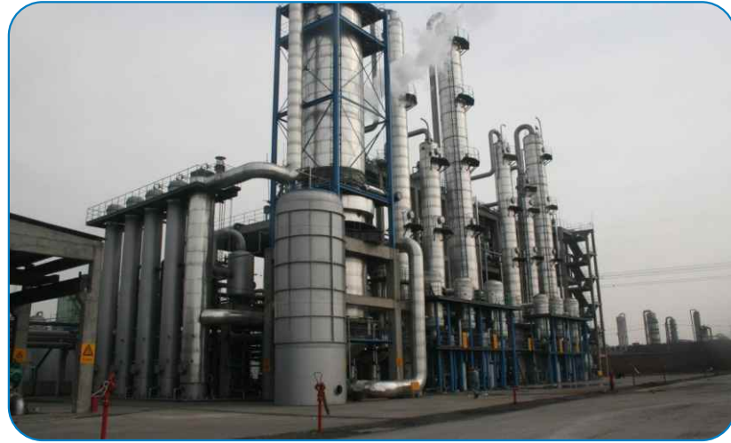
脱硫塔 Desulfurization tower
